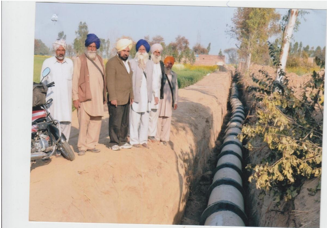
Pipeline at village Mahala Kalan
